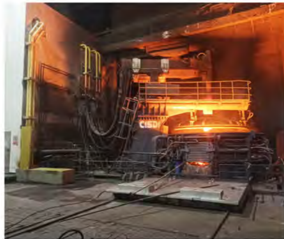
CISDI-AutoARC™, operating stably at the plant
