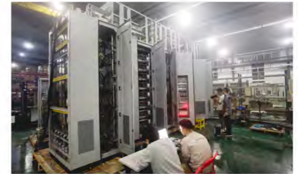
CISDI engineers implement ex-works testing for the installation of the IGBT unit at an EAF
