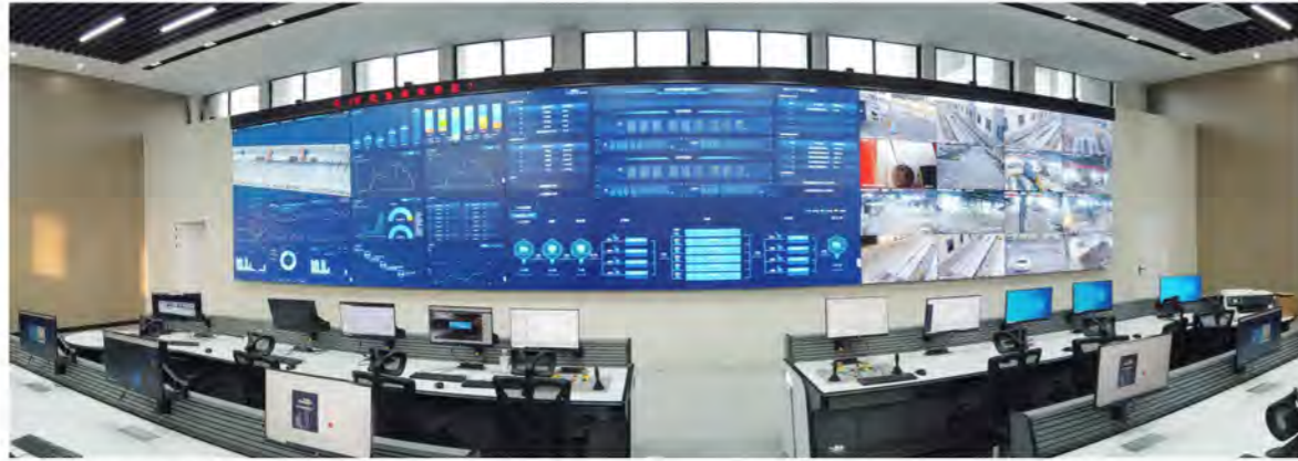
A wide-angle shot of the centralised control centre at Ouyeel's smart scrap plant
